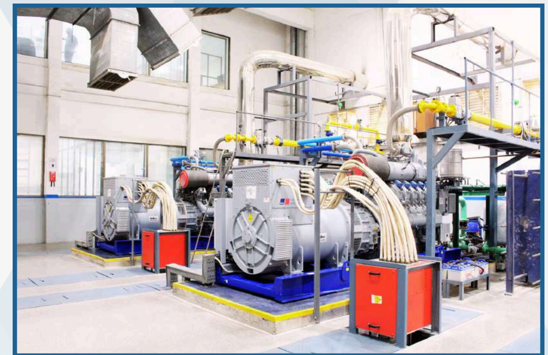
MTU 12V 40L64 Gas Generator (1521 KW)
