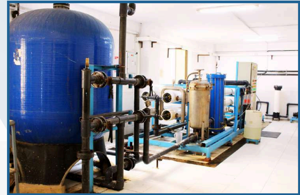
RO plant 120,000 gallon/day
