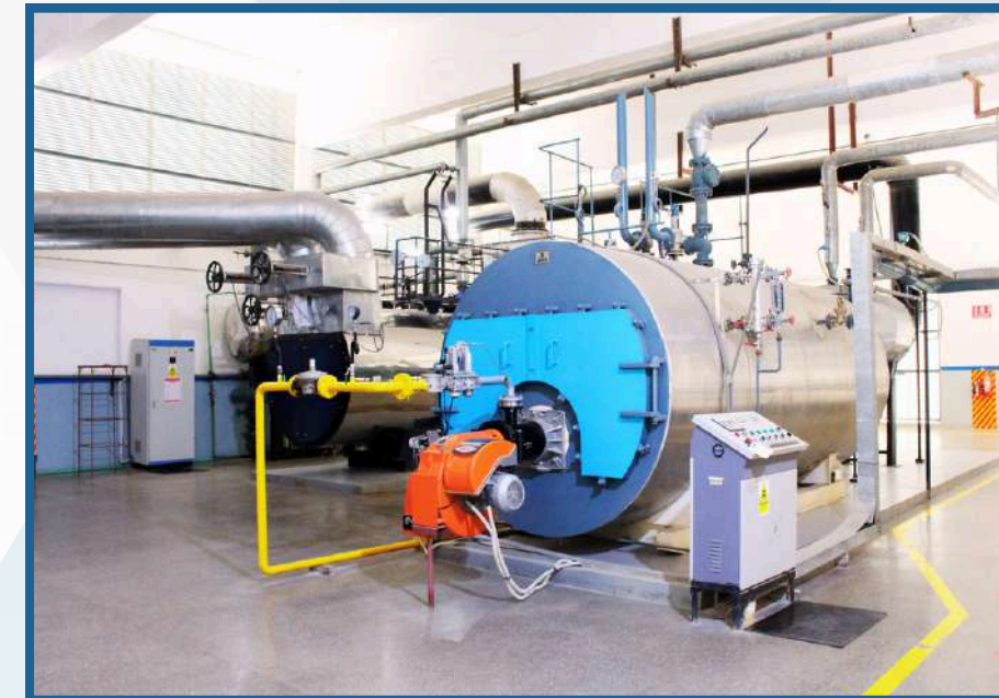
Gas fired boiler 4 Ton
