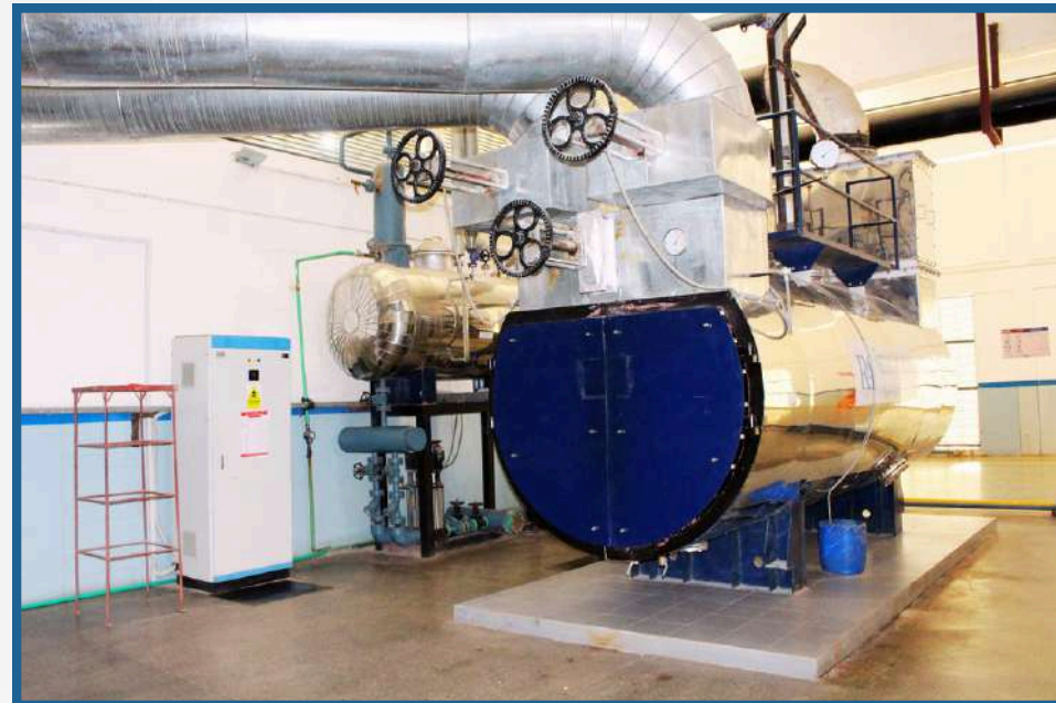
Waste heat recovery Boiler (WHRB) 1700 KG
